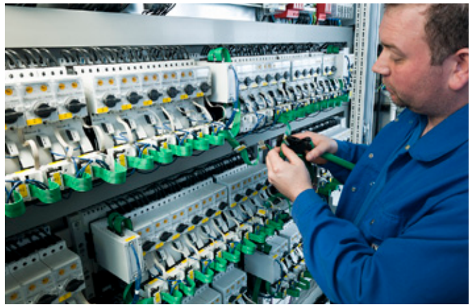
Around 500 Eaton PKE motor starters with a SmartWire-DT interface were used to control the exhaust air system.
