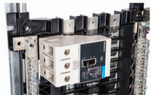
Example of Back-fed xGB Main breaker installed
