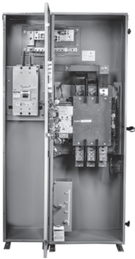
Separate Compartment for ATS and Breaker
