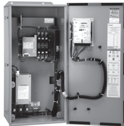
200 A ATS with ATC-300+ Controller
