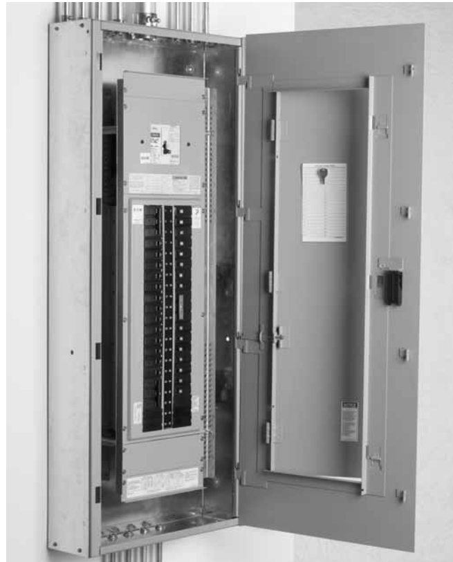
Trim Hanging on Surface Mounted Box
