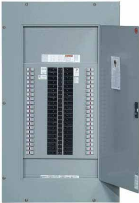
Type PRL1a Panelboard
