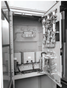
Mark V Field Controller
