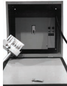
Breaker Test Cabinet
