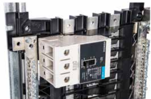
Example of Back-fed NGB Main breaker installed
