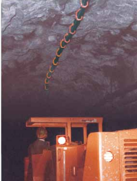
Bosserman Clips keep cables safely up and out of the way of moving equipment.
