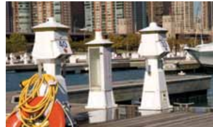
marine shore-power and dock lighting
