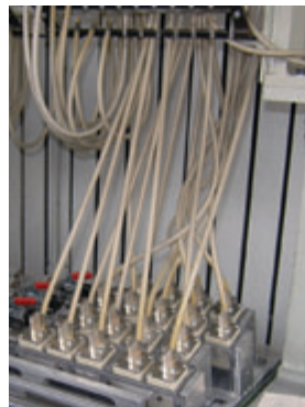
Fig. 3.8.2 – Sand filling for LV HRC fuse links
