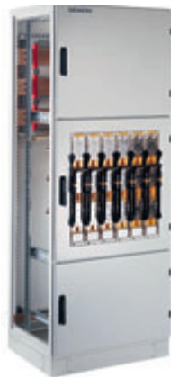
Fig. 3.3.3 – Distribution board with LV HRC in-line fuse switch disconnectors
