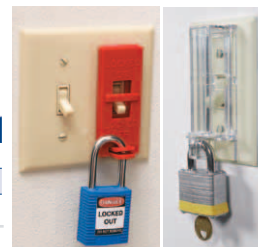
Wall Switch Lockouts
