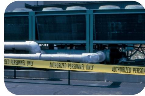
Visual barricading provides fast on-the-spot warning of potential danger.
